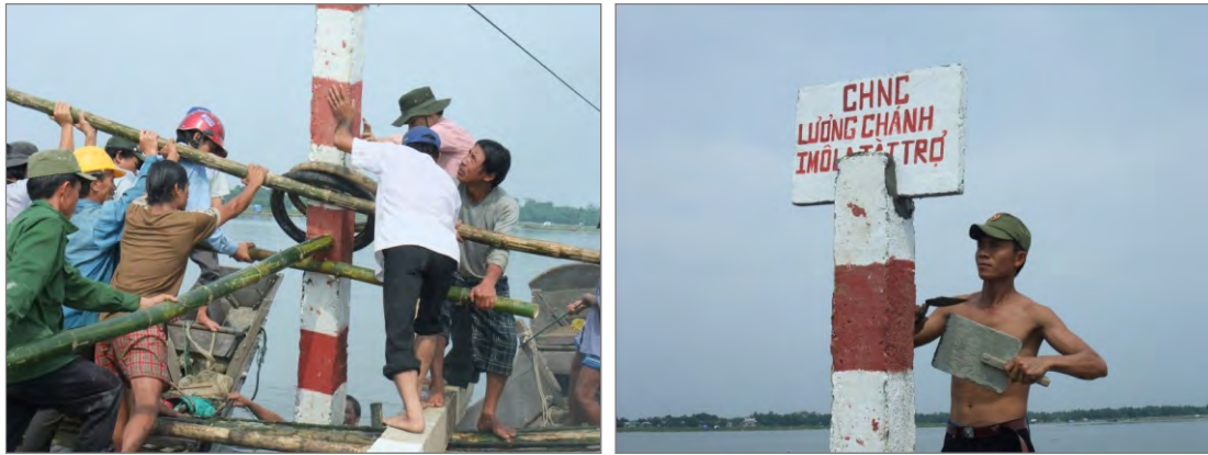
Figure 28 Concrete pole being installed for FA boundary demarcation by FAs in Loc Dien Commune
