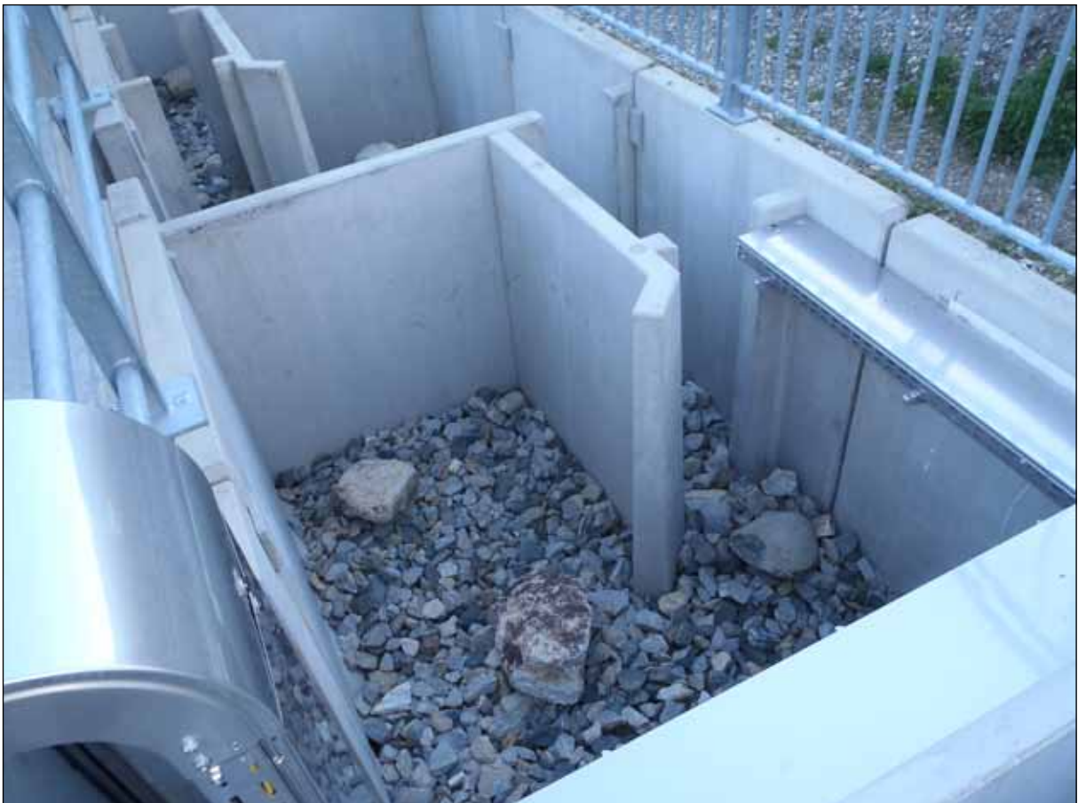
Figure 25: Example for coarse substrate in a fish pass (picture of vertical slot at hydropower plant Rottau River, Möll, Austria, picture by Friedrich T.)
