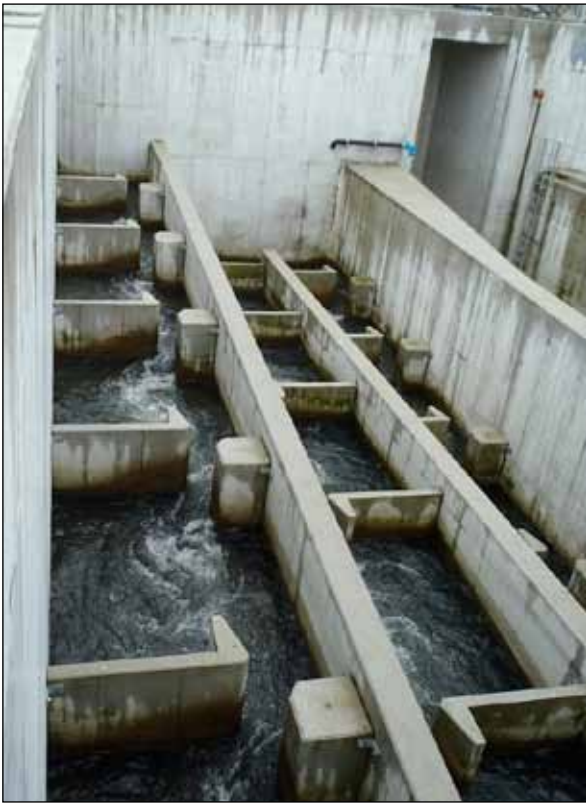
Figure 32: Vertical-slot fish pass at Greinsfurth Hydropower Plant on the River Ybbs (© Mielach)
