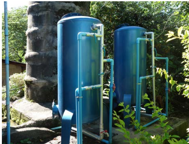
Water filtration system installed in Hae Ko and Huai Kang Pla villages, Chiang Rai Province, Thailand.
