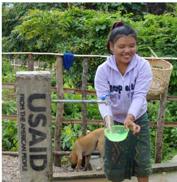
Villager in Ban Donkeo, Khammouan, Lao PDR draws water from one of five tap stands connected to nearly 4000 meters of pipeline and distribution lines installed by USAID Mekong ARCC .
