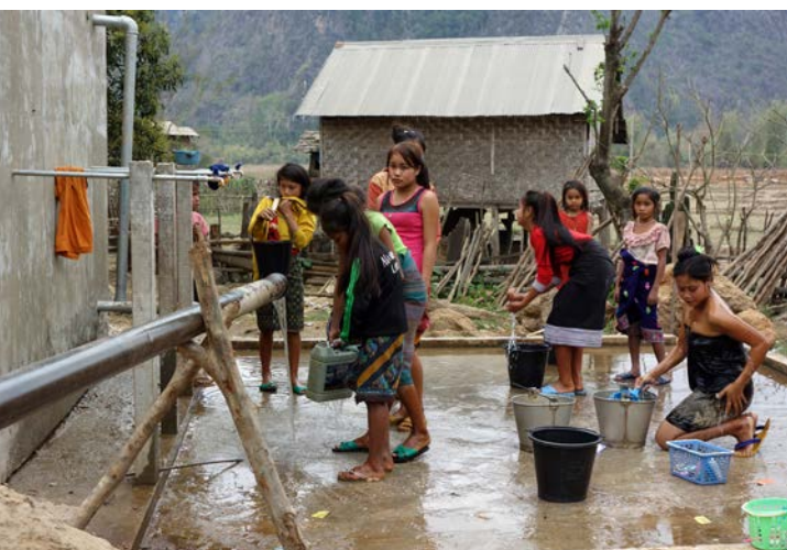
Women and girls of Ban Xong Village, Khammouan, Lao PDR collect water and bathe in the evening from the newly constructed water tank and piping.
