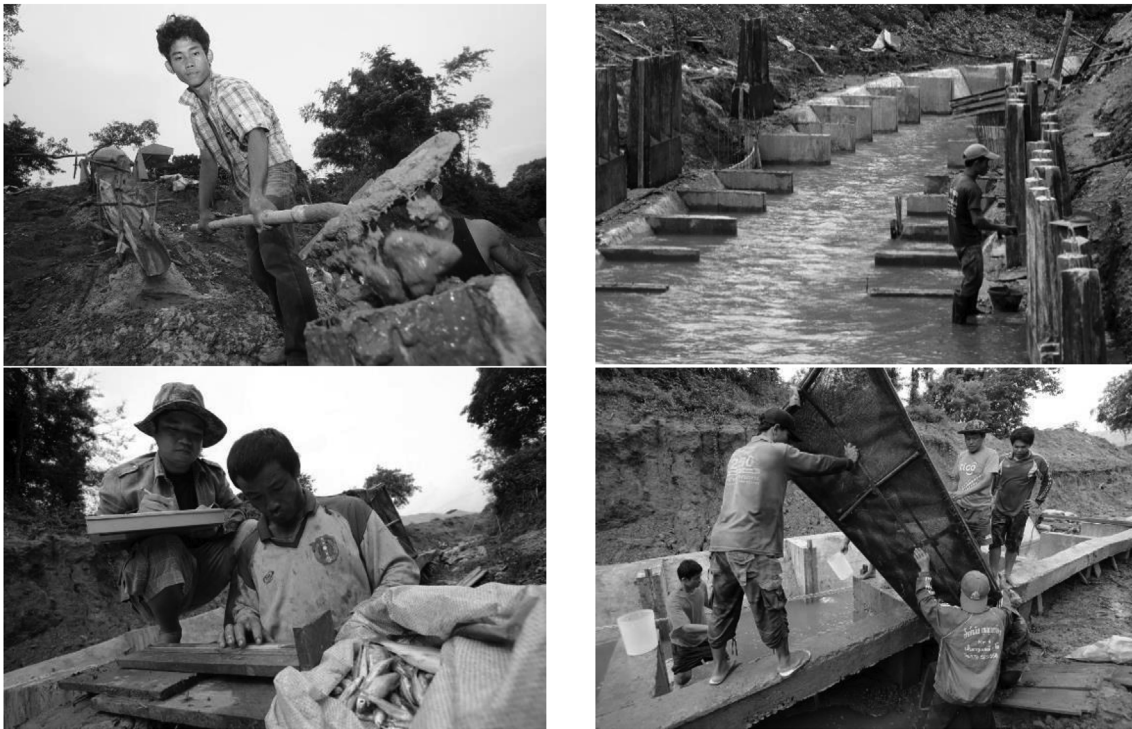
Fig. 4. Engaging in construction (top) and monitoring (bottom) of Pak Peung fishway and regulator was an important component of project success (Photos courtesy of Jim Holmes).
